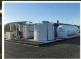
ECT2 Patented Resin Regeneration Facility
