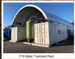
FTA Water Treatment Plant
