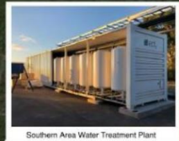
Southern Area Water Treatment Plant
